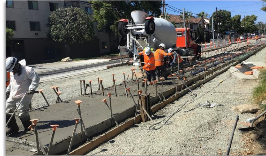
Embedded Track - Santa Ana Blvd & Lacy St
