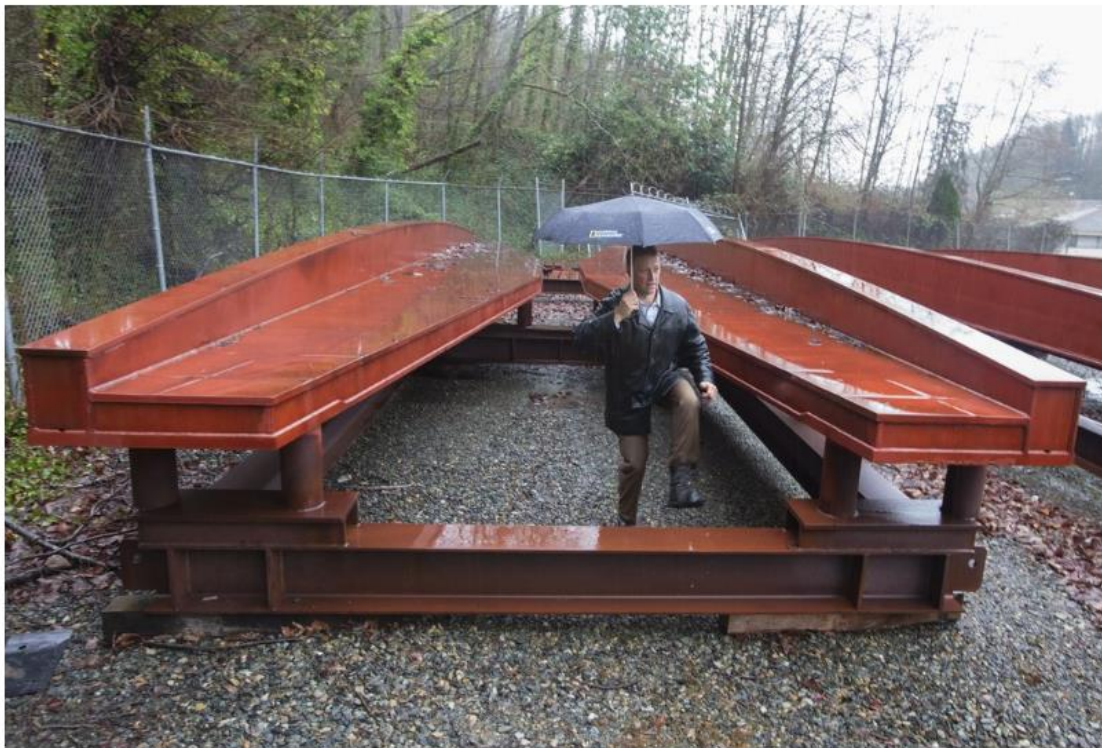
John Sleavin, a senior technical director at Sound Transit, walks out from the track bridge system that will transition the light-rail track from Interstate 90's fixed span to the floating-bridge span. (Steve Ringman/The Seattle Times)
