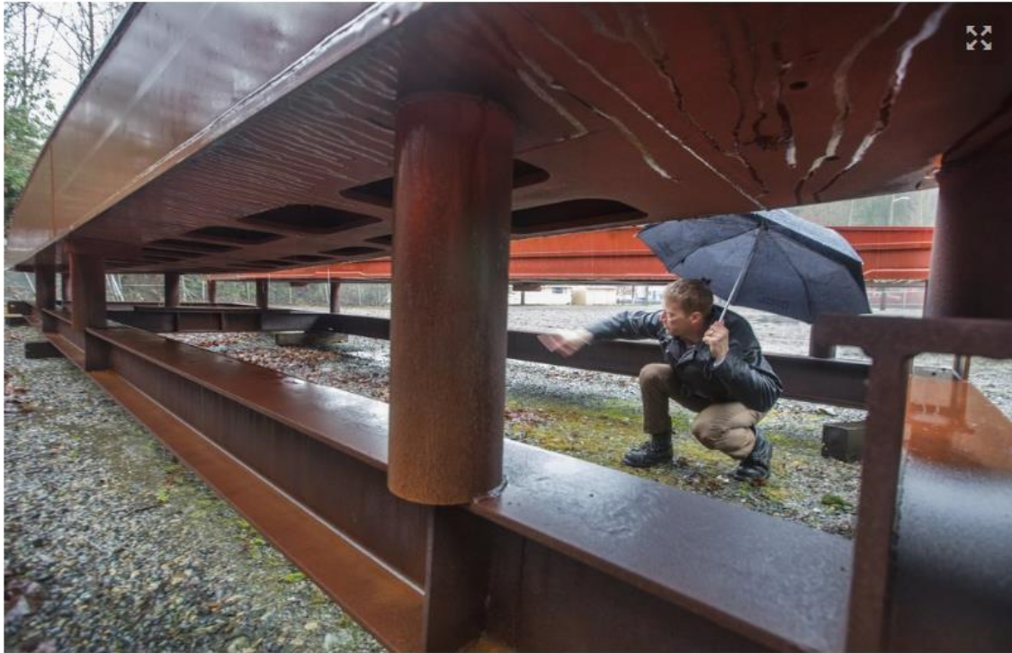
John Sleavin, a senior technical director at Sound Transit, looks at the track bridge system that will transition the light-rail track from I-90's fixed span to the floating-bridge span. (Steve Ringman/The Seattle Times)
